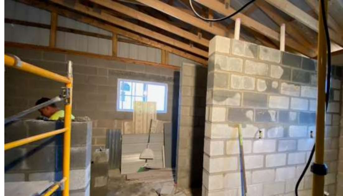
Apr 1 – JJ Wickard, Wyatt Heller and Steve Steffel work on supplying block and mortar mix.
