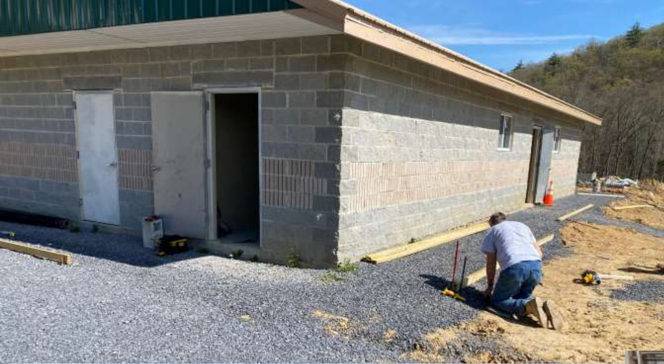
April 23, 2024 Ron Adlesic and Steve Steffel add forms for concrete and pour a concrete countertop for one of four – 3 sink units.
